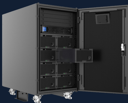
Single-phase 6-10 kVA UPS with 8 x 40/50Ah battery modules and no PDM
